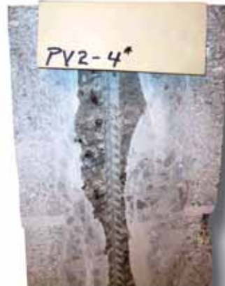
Cross section of blockwall cell illustrating improper vibration technique
